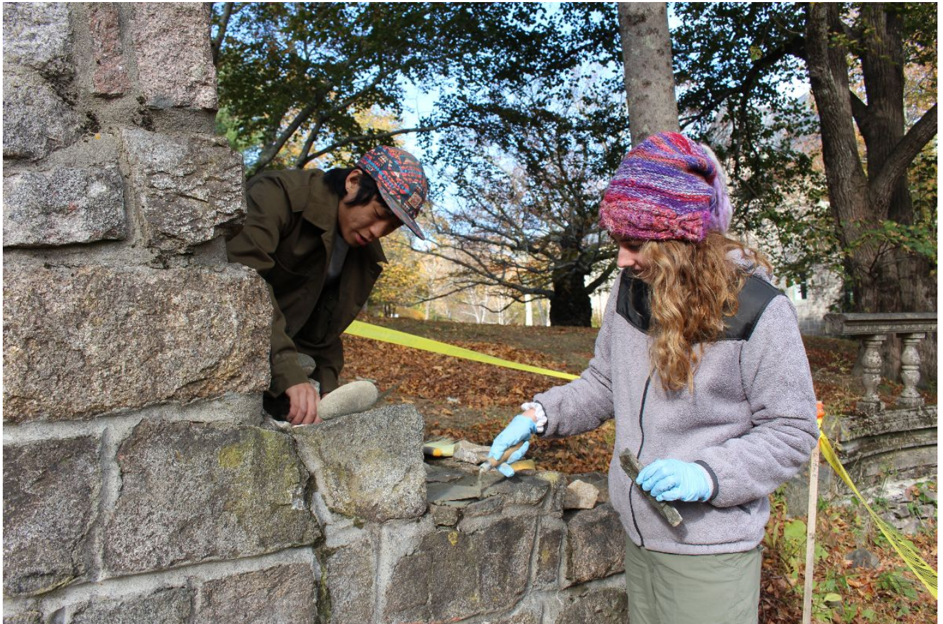
COA students Max Lee and Teaghan Rose take part in the restoration of the more-than-a-century-old stone arch at the school's sunken garden. PHOTO COURTESY OF COA
